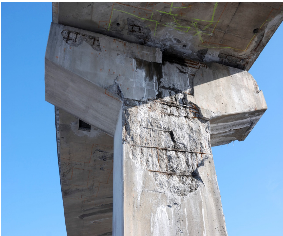
1-rasm. Ko‘prik ustunini muqobil muzdan tushirishdan beton yuzani yo‘qolishi
